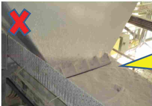
Opening / Crack in Chute
