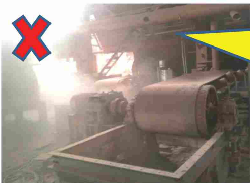
Discharge Hood not boxed back
