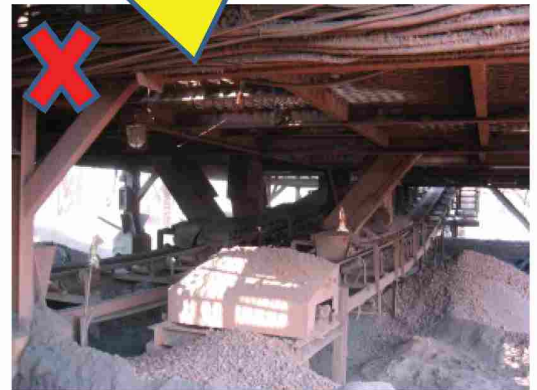
Grated flooring causing pile up below
